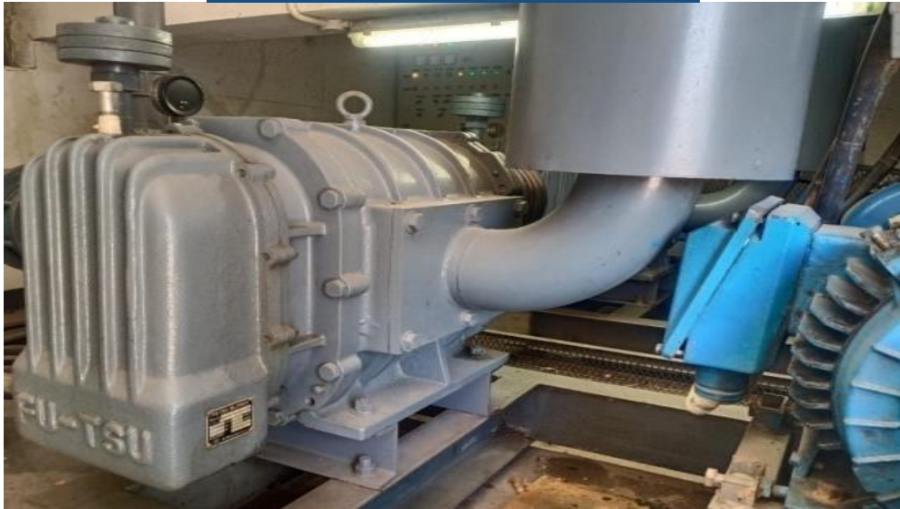
Blower Pump STP
