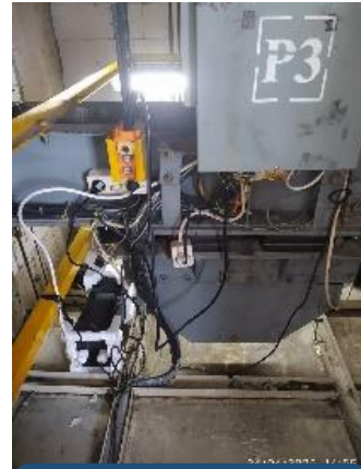
Emergency Lamp R. Lift
